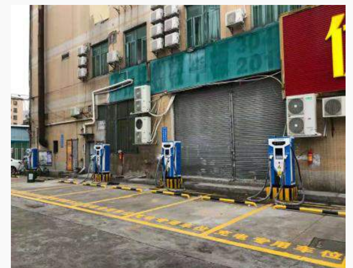
Foshan Nanhai charging station
