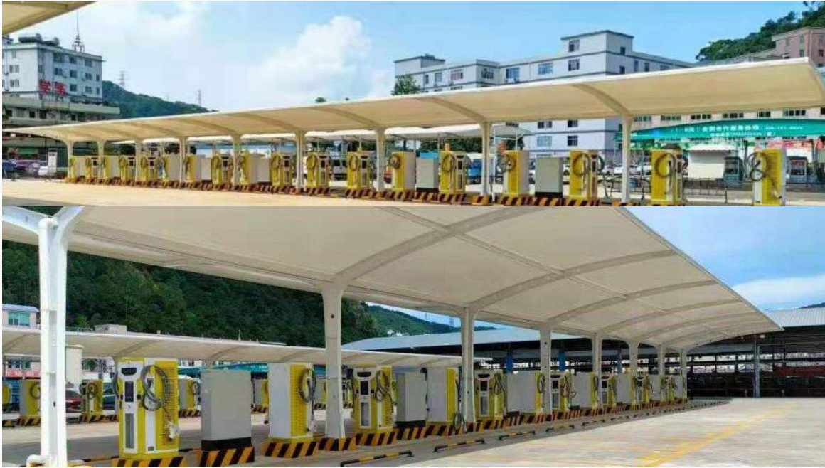
Guangzhou Taibang logistics charging station
