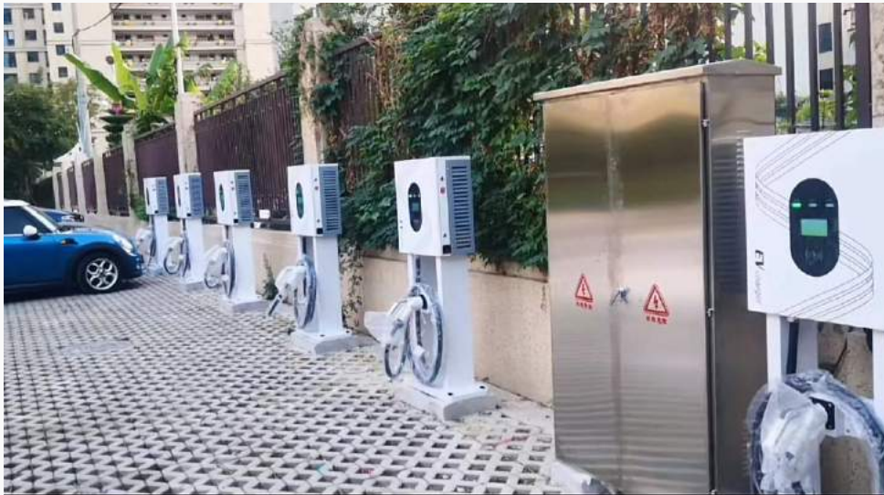
Ningbo charging station
