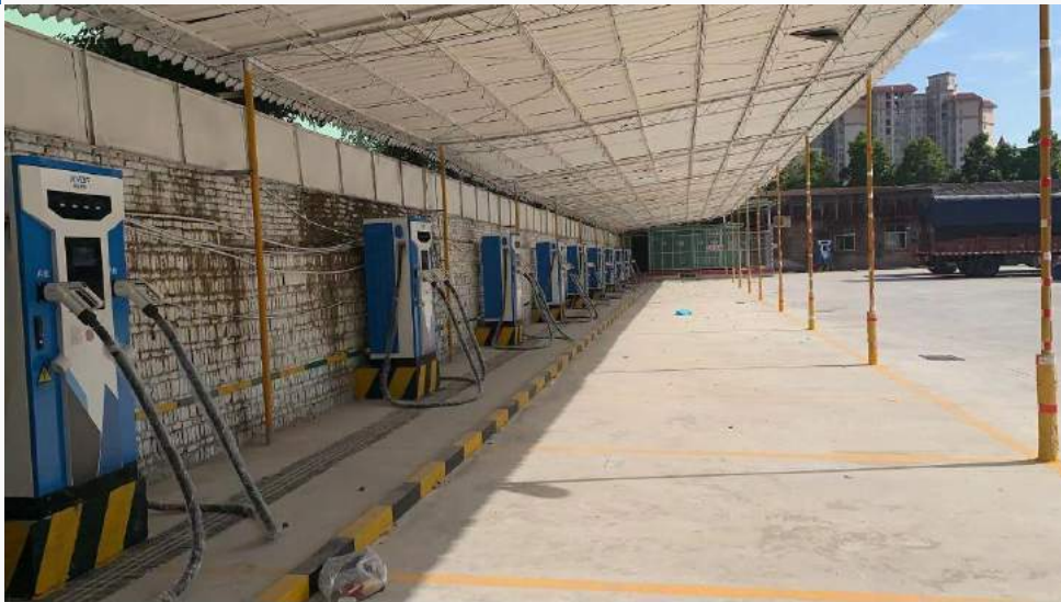
Ningbo charging station
