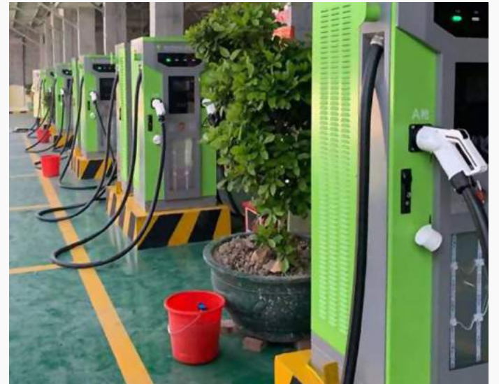
Shanwei Zhongwo charging station
