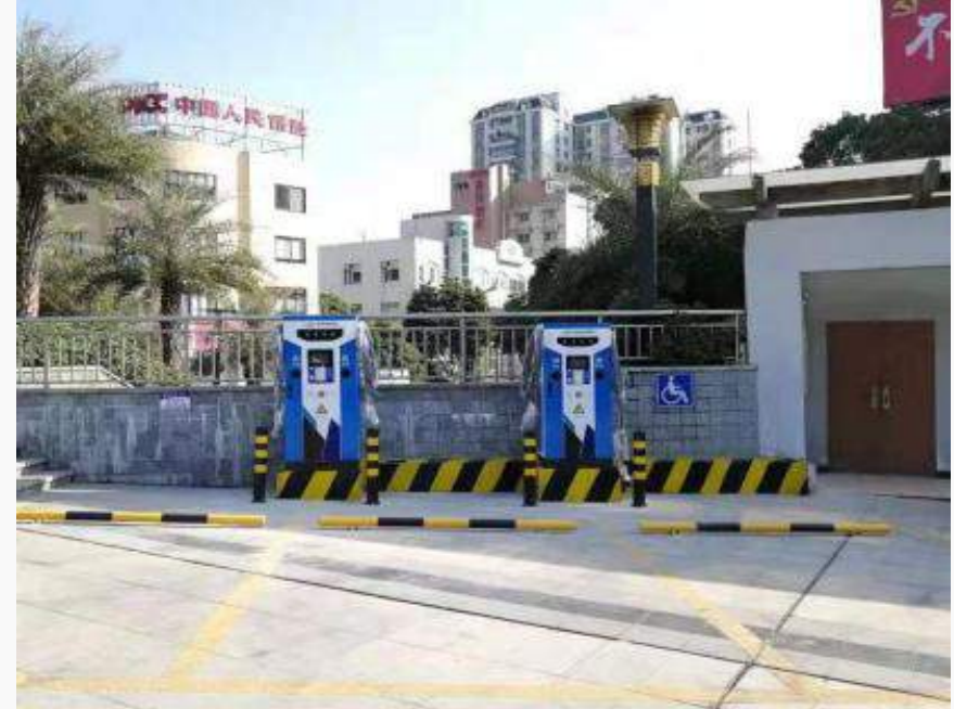
Foshan Nanhai charging station
